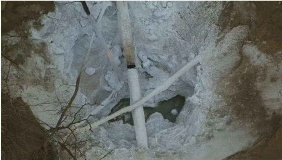
Figure 3: CO 2 leakage from the rupture of a Denbury Resources CO 2 pipeline in Yazoo County Mississippi, USA 22 February 2020 [16]
